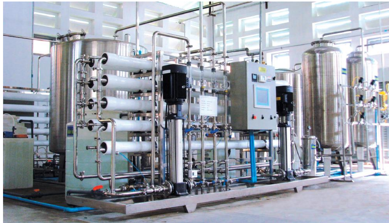
(哈萨克斯坦)阿拉木图市ALPHARMACHIM制药厂 3m 3 /h二级反渗透纯化水系统 3m 3 /h two-stage reverse osmosis purified water system of ALPHARMACHIM Pharmaceutical Factory,Alma-Ata, Kazakhstan
