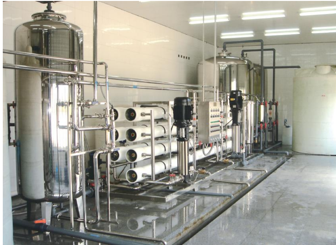
黑龙江摇篮乳业股份有限公司 15m 3 /h二级反渗透纯化水系统 15m 3 /h two-stage reverse osmosis purified water system of Heilongjiang Yaolan Dairy Co., Ltd.
